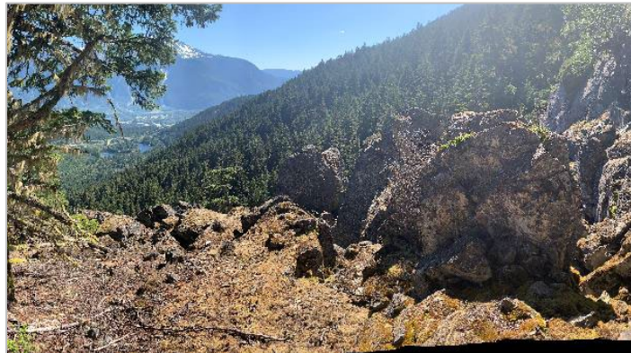
Photo 17. Heavily dilated unstable rock masses on Jason Creek, toppling to the left towards the creek. Photo: July 22, 2022.
