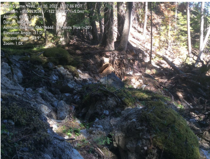
Photo 15. Unstable slope on Jason Creek sidewall. Photo: July 20, 2022.
