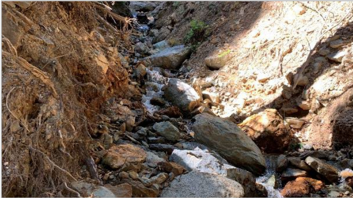
Photo 7. Jason Creek mid section, both valley sides are moving inwards due to deep-seated landsliding. Photo: July 22, 2022.
