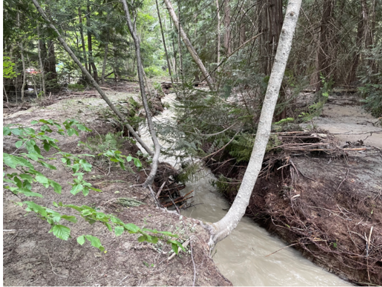
Figure 21 – Looking Downstream Along Previous Constructed Ditch now Incised Upstream of New Place Creek Outlet into Gates Lake
