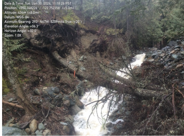
January 30, 2024. Two trees have fallen, but otherwise bank failure has not grown.
