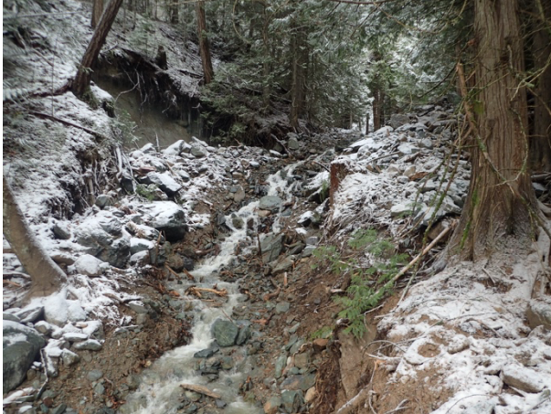
Dec 12, 2021. Right bank erosion site, just above Reid Road. Waypoint 2, Appendix 1.
