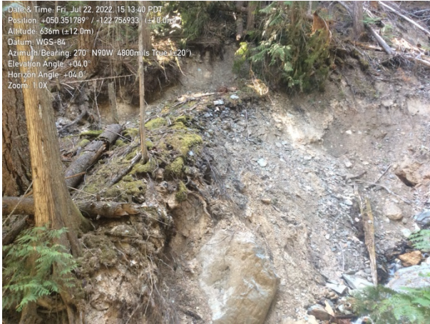
July 22, 2022. Slump on right bank below main failure site. Waypoint 15, Appendix 1.
