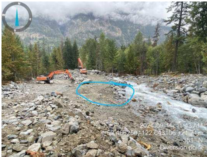
Image 5: diversion point circled in blue (2024-09-11 11:43 AM)
