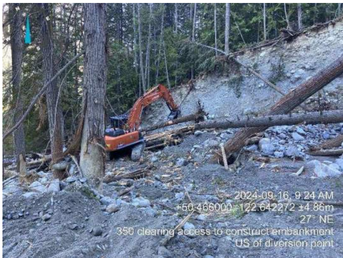
Image 2: 350 excavator moving fallen trees to establish access to construct the embankment (2024-09-16 9:24 AM)
