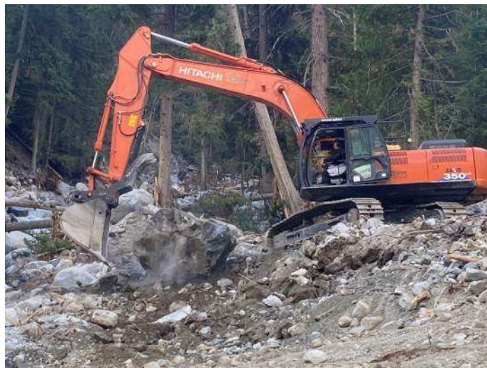
Image 3: 350 excavators moving large boulder to prevent flow from impinging on the embankment (2024-09-09 @ 10:04 AM)
