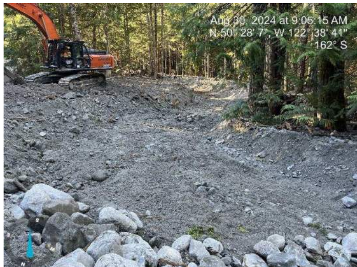
Image 8: 350 excavator sorting through excavated materials to stockpile large boulders for riprap armoring (2024-08-30 @ 9:05 AM)
