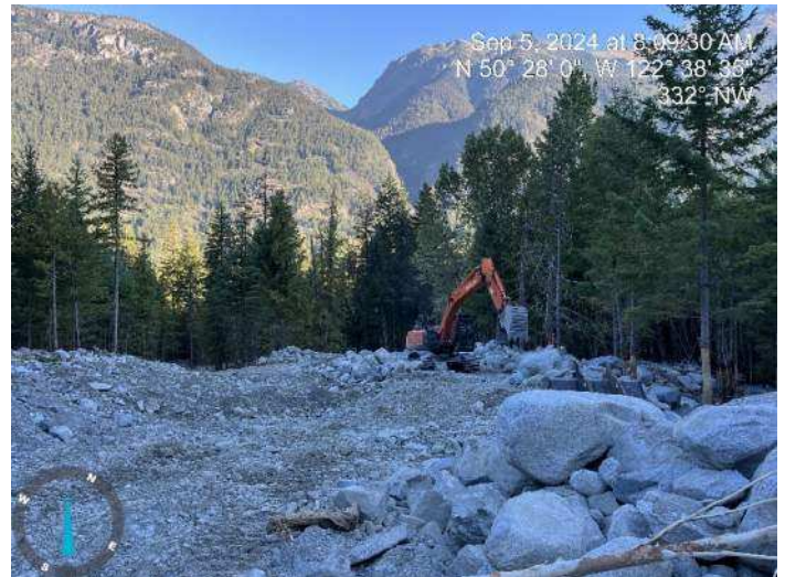
Image 7: 210 excavator continued sorting through excavated materials to build up the proposed embankment (2024-09-05 @ 8:09 AM)
