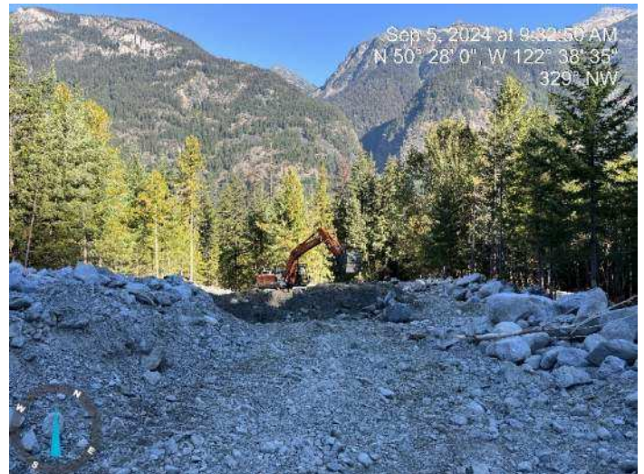
Image 11: 210 excavator continued sorting through excavated materials to build up the proposed embankment (2024-09-05 @ 9:32 AM)
