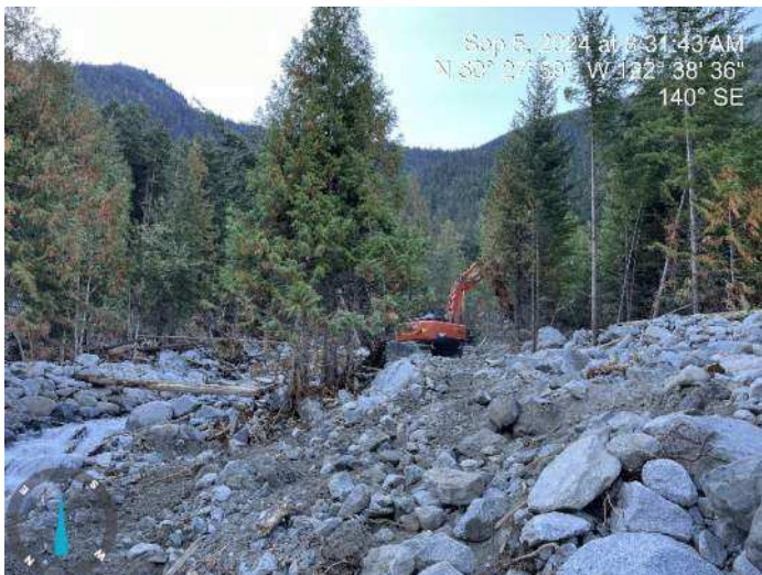
Image 8: 350 excavator was removing fallen trees and relocating rocks to create an access road (2024-09-05 @ 8:31 AM)
