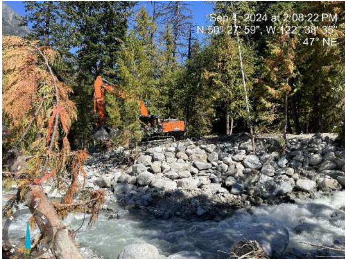
Image 18: 350 excavator sorting through materials from the debris flood deposits to build up the proposed embankment (2024-09-04 @ 2:08 PM)
