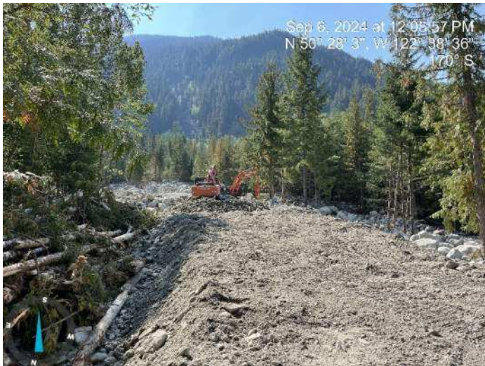
Image 12: 350 and 210 excavators working together to excavate proposed channel, and stockpile materials to build up the proposed embankment (2024-09-06 @ 12:05 PM)
