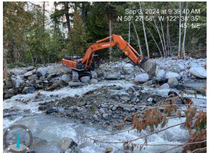
Image 5: 350 excavator relocating boulders within the existing channel to block off the side channel hugging the left bank (looking upstream) (2024-09-03 9:39 AM)
