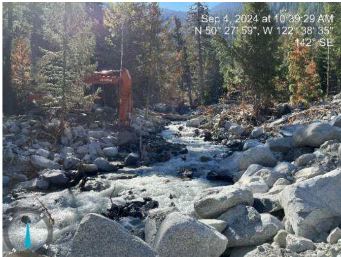
Image 12: 350 excavator continued to reinforce the toe of the proposed embankment along the left bank (looking upstream) (2024-09-04 @ 10:39 AM)
