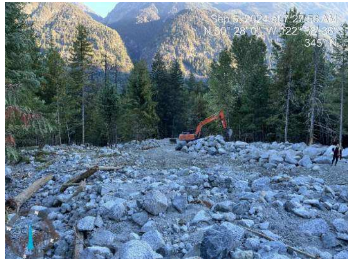
Image 3: 210 excavator started sorting through excavated materials to build up the proposed embankment (2024-09-05 @ 7:27 AM)
