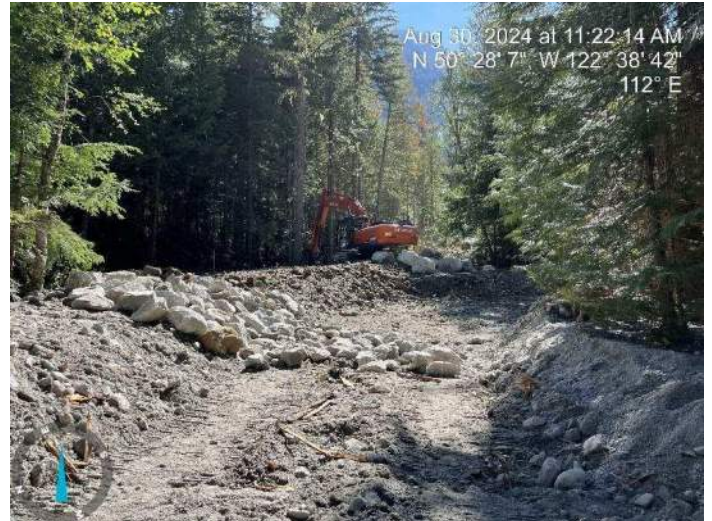
Image 11: 350 excavator continued to sort through excavated materials to find large boulders for riprap armoring (2024-08-30 @ 11:22 AM)
