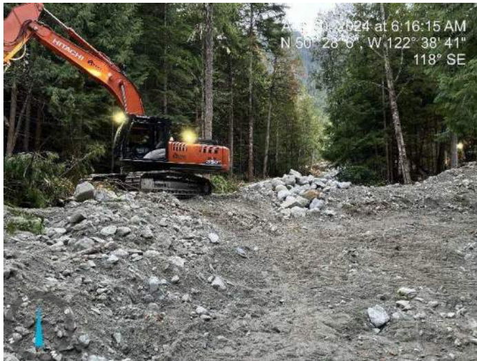
Image 2: 350 excavator sorting through excavated materials to stockpile large boulders for riprap armoring (2024-08-30 6:16 AM)
