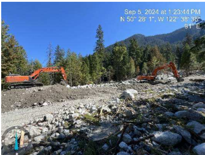
Image 20: 210 excavator continued sorting through excavated materials to build up the proposed embankment. 350 excavator started excavating the proposed channel (2024-09-05 @ 1:23 PM)
