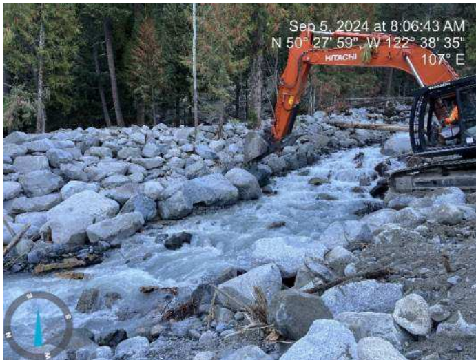
Image 6: 350 excavator continued reinforcing the toe of the proposed embankment along the left bank (looking upstream) of the existing channel (2024-09-05 @ 8:06 AM)
