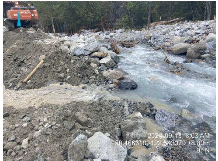
Image 3: Water in Place Creek beginning to flow into the reestablished channel (2024-09-13 @ 8:03 AM)
