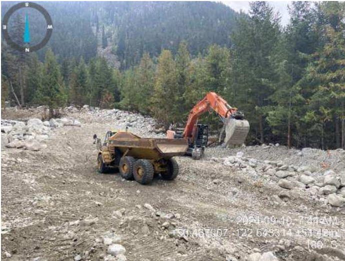
Image 2: 350 excavator loading rock truck with boulders to be used to armour embankment (2024-09-10 7:44 AM)
