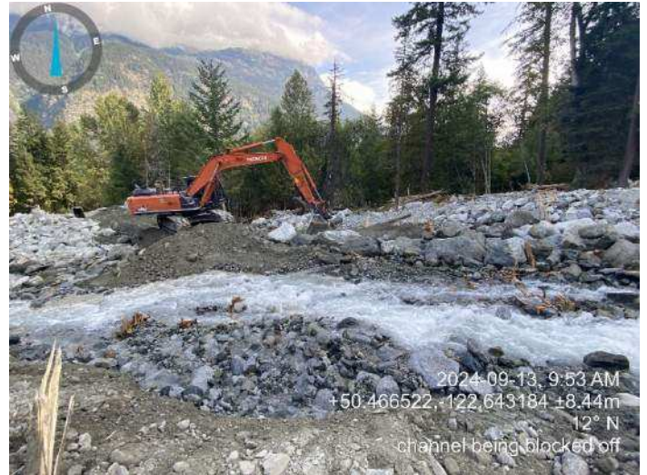
Image 7: 350 excavator blocking off the former channel with 100% flow in the reestablished channel (2024-09-13 @ 9:53 AM)
