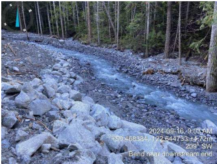
Image 6: Channel bank armoring in this area not impacted by higher flows over the weekend (2024-09-13 @ 9:16 AM)
