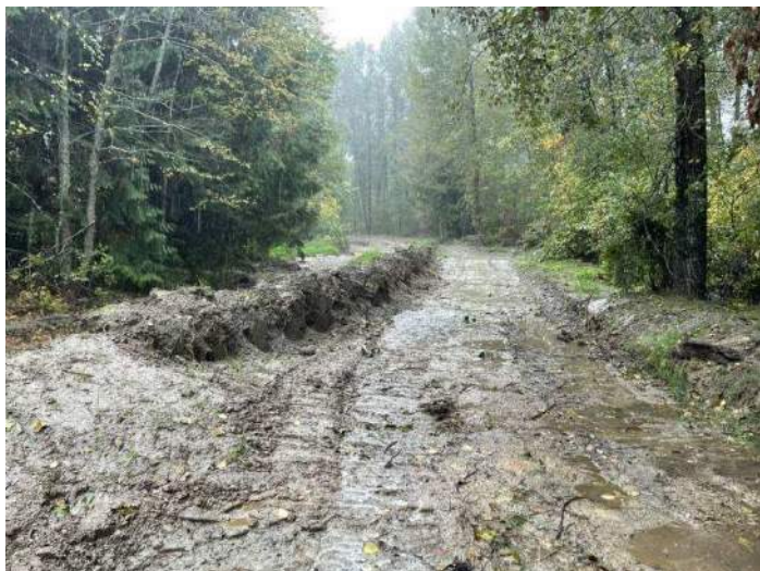
Image 1: Fill from gabion baskets left piled along emergency ditch top of bank (looking west)(2024-09-25)
