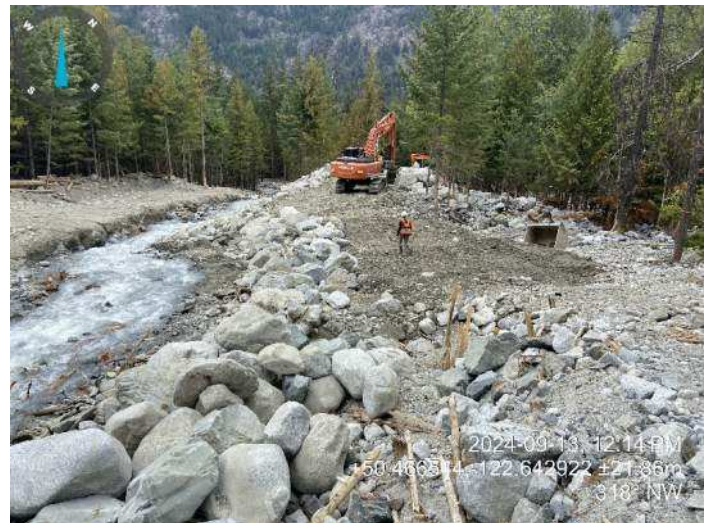
Image 9: 350 excavator grading the embankment near the diversion point after all flow has been diverted (2024-09-13 @ 12:14 PM)
