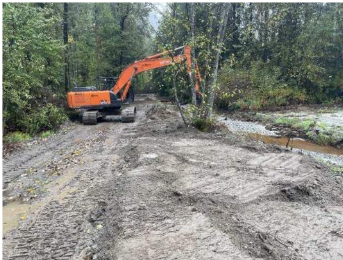
Image 4: Ongoing removal of piled fill at time of Stantec departure from site (looking east) (2024-09-25)
