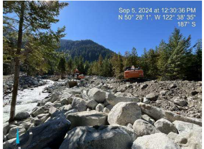
Image 19: 210 excavator continued sorting through excavated materials to build up the proposed embankment. 350 excavator continued to widen the right bank of the existing channel (2024-09-05 @ 12:30 PM)
