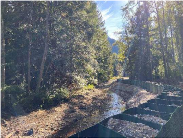
Image 10: Low flow from groundwater seepage in the diversion ditch (2024-09-16 @ 15:38 AM)
