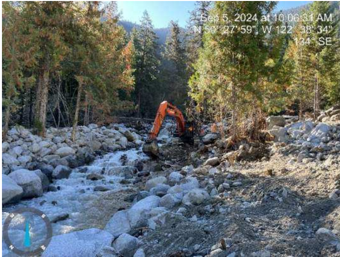
Image 14: 350 excavator started to widen the right bank of the existing channel (2024-09-05 @ 10:06 AM)
