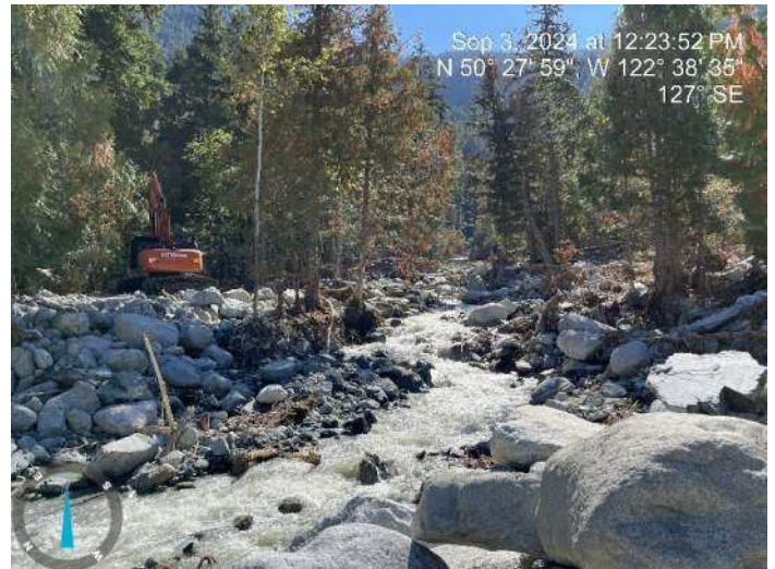
Image 9: 350 excavator proceeded to source materials from the debris flood deposits to build up the proposed ermbankment (2024-09-03 @ 12:23 PM)
