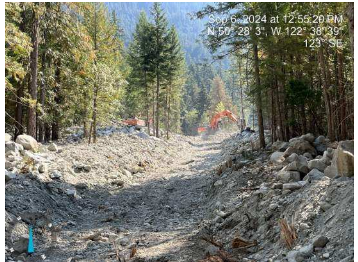
Image 13: 350 and 210 excavators working together to excavate proposed channel, and stockpile materials to build up the proposed embankment (2024-09-06 @ 12:55 PM)
