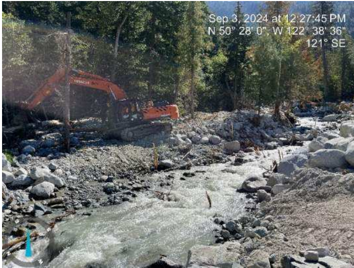
Image 10: 350 excavator proceeded to source materials from the debris flood deposits to build up the proposed embankment (2024-09-03 @ 12:23 PM)
