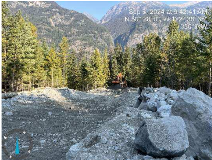
Image 6: 350 and 210 excavators working together to excavate proposed channel, and stockpile materials to build up the proposed embankment (2024-09-06 @ 9:42 AM)
