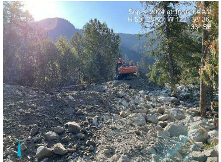
Image 7: 210 excavator continued to stockpile materials to build up the proposed embankment while 350 excavator was out of service (2024-09-06 @ 10:02 AM)
