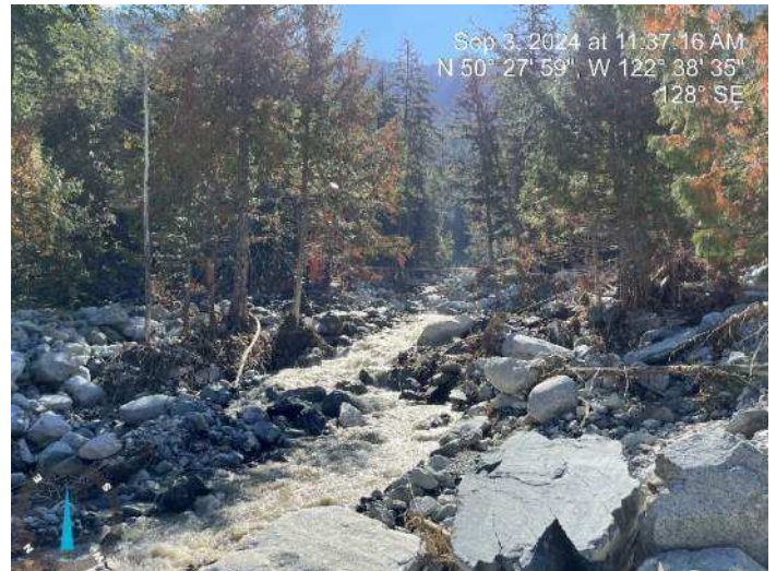
Image 7: 350 excavator completed blocking the side channel that was along the left bank (looking upstream) (2024-09-03 @ 11:37 AM)
