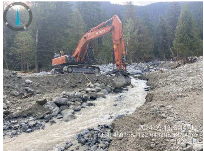
Image 5: 350 excavator adding boulders to the channel bank at the diversion point (2024-09-13 @ 8:44 AM)
