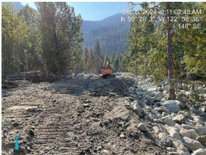
Image 8: 210 excavator continued to stockpile materials to build up the proposed embankment while 350 excavator was out of service (2024-09-06 @ 11:02 AM)
