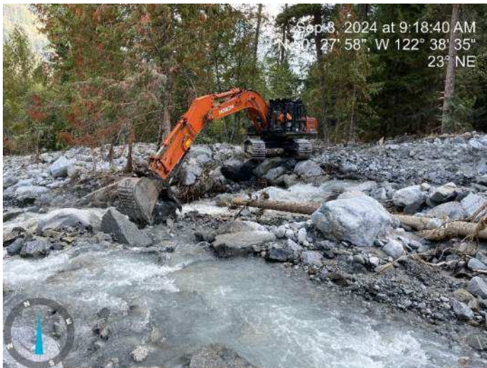
Image 4: 350 excavator relocating boulders within the existing channel to block off the side channel hugging the left bank (looking upstream) (2024-09-03 9:18 AM)
