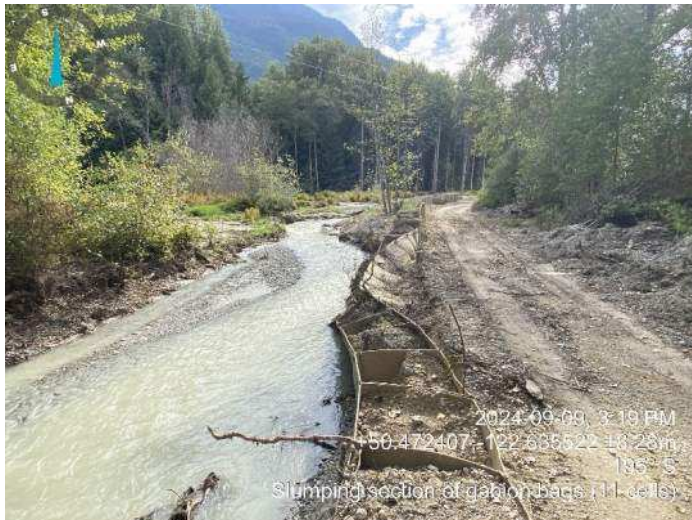
Image 8: Approximately 11 gabion bags have slumped into the drainage ditch, just downstream of the edge of the hydro corridor. (2024-09-09 @ 3:19 PM)
