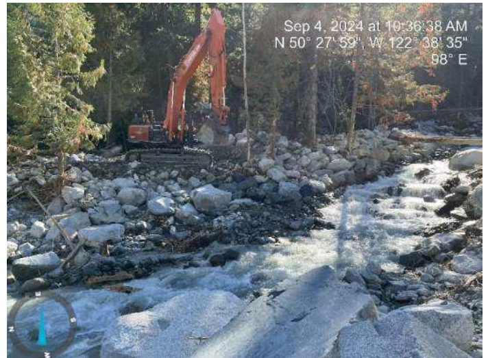
Image 11: 350 excavator continued to reinforce the toe of the proposed embankment along the left bank (looking upstream) (2024-09-04 @ 10:36 AM)
