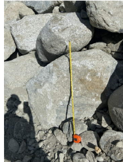
Image 7: typical size of large boulders at base of channel bank armouring. 1.0 m tape measure for scale. (2024-09-09 @ 12:56 PM)
