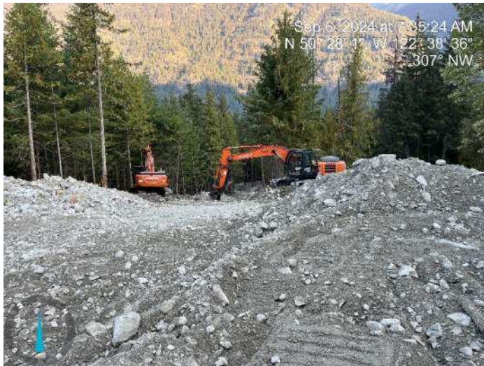
Image 2: 350 and 210 excavators working together to excavate proposed channel, and stockpile materials to build up the proposed embankment (2024-09-06 7:35 AM)
