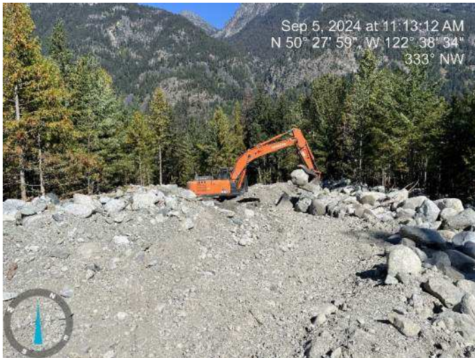
Image 16: 210 excavator continued sorting through excavated materials to build up the proposed embankment (2024-09-05 @ 11:13 AM)
