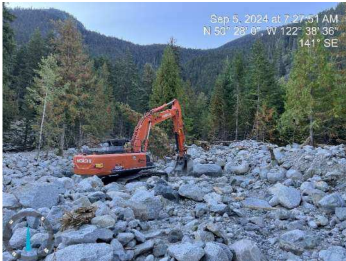
Image 2: 350 excavator relocating rocks and removing fallen trees to create an access road (2024-09-05 7:27 AM)
