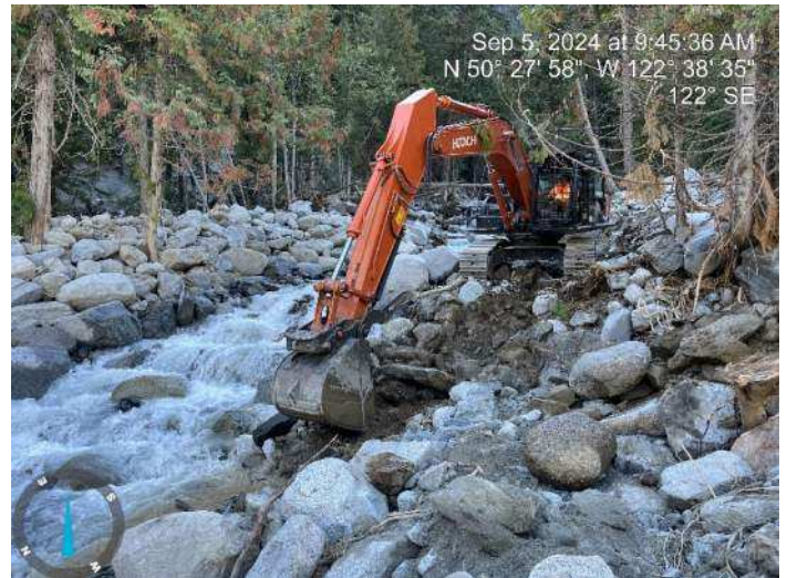
Image 13: 350 excavator started to widen the right bank of the existing channel to promote water towards the orientation of the proposed channel (2024-09-05 @ 9:45 AM)
