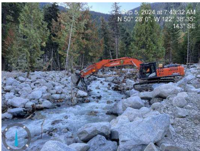
Image 4: 350 excavator started reinforcing the toe of the proposed embankment along the left bank (looking upstream) of the existing channel (2024-09-05 7:43 AM)
