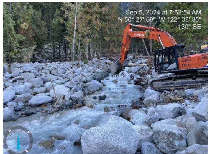
Image 5: 350 excavator started reinforcing the toe of the proposed embankment along the left bank (looking upstream) of the existing channel (2024-09-05 7:52 AM)
