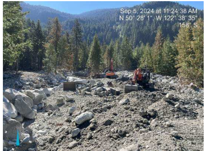
Image 17: 210 excavator continued sorting through excavated materials to build up the proposed embankment. 350 excavator continued to widen the right bank of the existing channel (2024-09-05 @ 11:24 AM)
