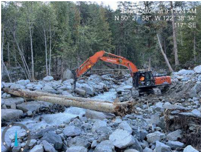
Image 10: 350 excavator was reinforcing the toe of the proposed embankment along the left bank (looking upstream) of the existing channel (2024-09-05 @ 9:13 AM)
