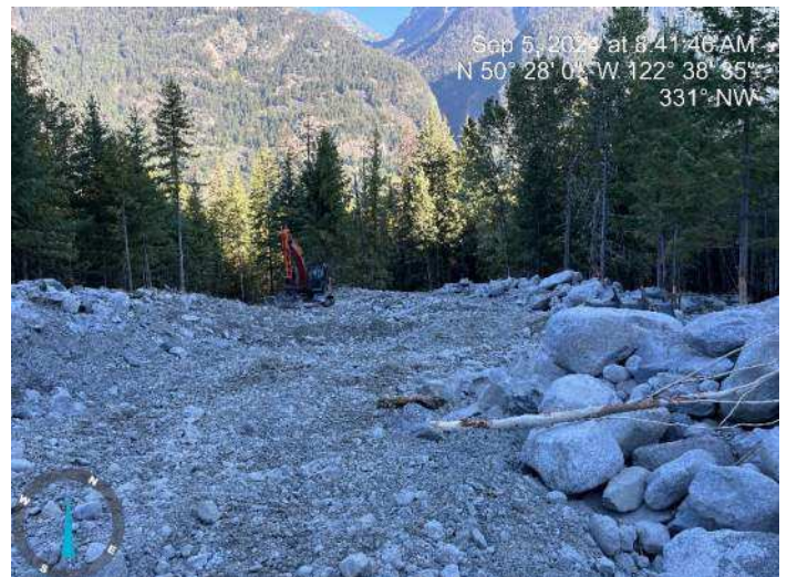
Image 9: 210 excavator continued sorting through excavated materials to build up the proposed embankment (2024-09-05 @ 8:41 AM)
