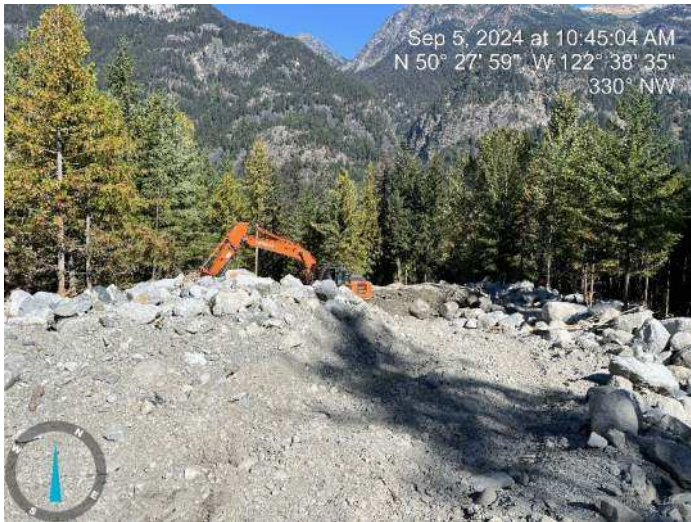
Image 12: 210 excavator continued sorting through excavated materials to build up the proposed embankment (2024-09-05 @ 10:45 AM)
