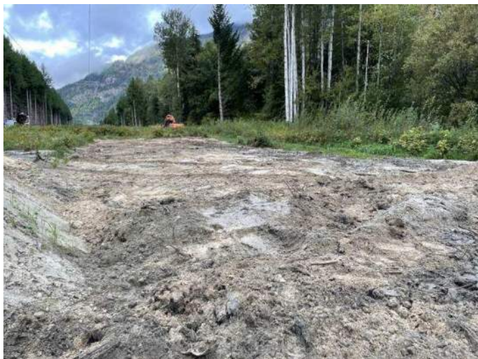
Image 1: Upstream extent of emergency ditch filled in with emergency bank material (looking west)(2024-09-23)
