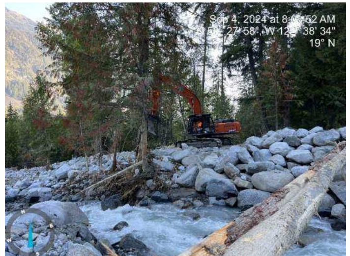
Image 5: 350 excavator continued to build up the proposed embankment along the left bank (looking upstream) of the current Place Creek channel (2024-09-04 8:08 AM)
