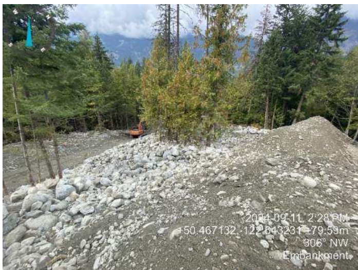
Image 6: embankment immediately downstream of diversion point (2024-09-11 @ 2:28 PM)
