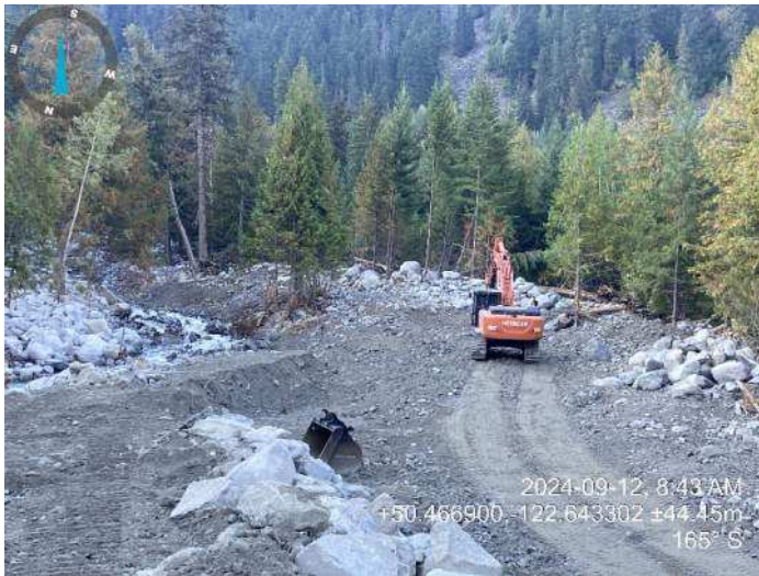
Image 2: 310 excavator removing surplus material from left (west) channel bank to be used to build the embankment (2024-09-12 8:43 AM)
