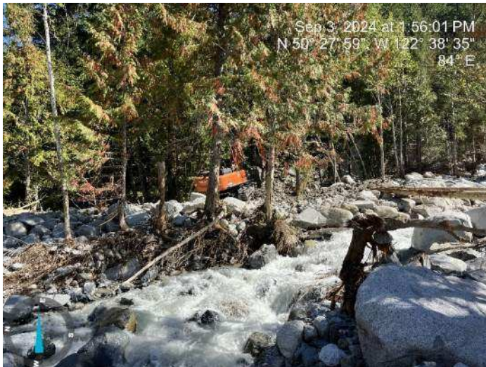
Image 12: 350 excavator continued to source materials from the debris flood deposits to build up the proposed embankment (2024-09-03 @ 1:56 PM)
