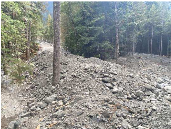
Image 2: material dumped by rock truck prior to being shaped and compacted (2024-09-11 6:55 AM)
