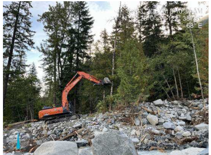
Image 3: 350 excavator clearing trees along the left bank of Place Creek channel where the proposed embankment will be built (2024-09-03 @ 8:10 AM)
