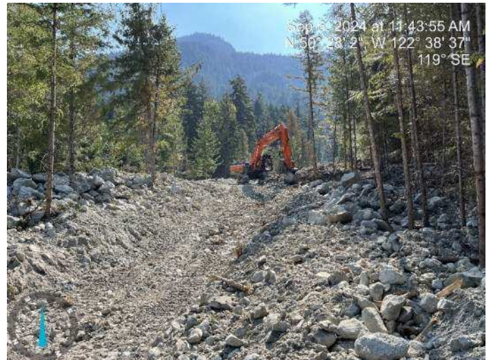
Image 11: 350 excavator started to excavate the proposed channel after being temporarily out of service from 9:55 AM – 11:38 AM (2024-09-06 @ 11:43 AM)
