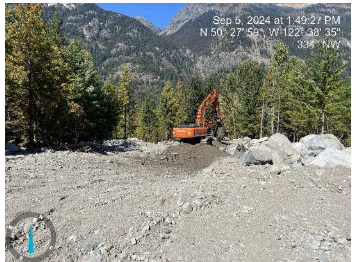
Image 21: 210 excavator continued sorting through excavated materials to build up the proposed embankment. 350 excavator continued excavating the proposed channel (2024-09-05 @ 1:49 PM)
