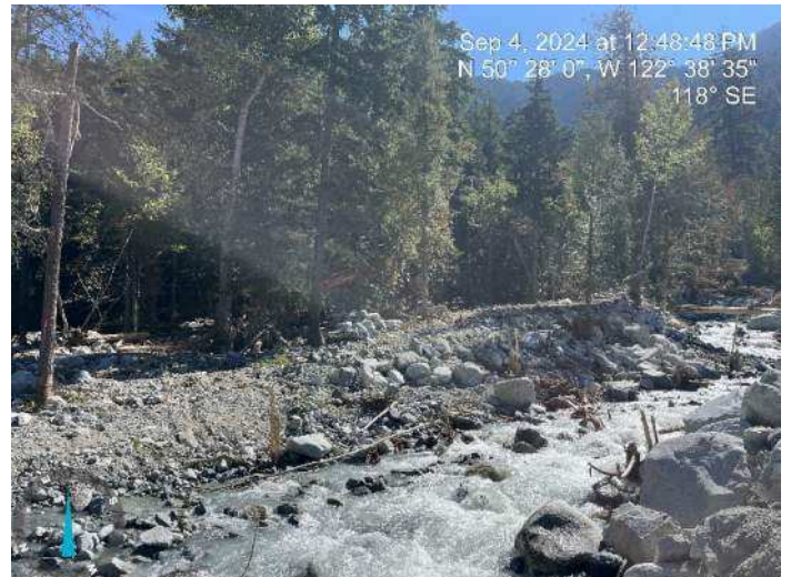
Image 17: 350 excavator sorting through materials from the debris flood deposits to build up the proposed embankment (2024-09-04 @ 12:48 PM)
