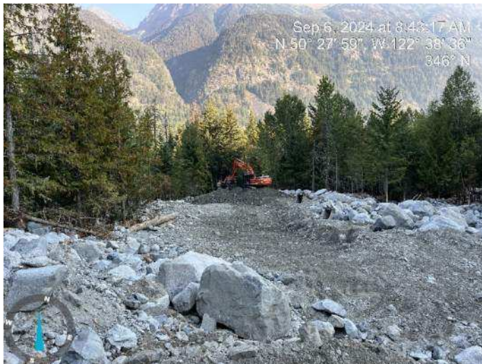
Image 4: 350 and 210 excavators working together to excavate proposed channel, and stockpile materials to build up the proposed embankment (2024-09-06 8:43 AM)
