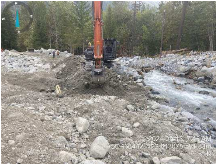
Image 2: 310 excavator removing material to begin diverting flow into the reestablished channel (2024-09-13 7:45 AM)
