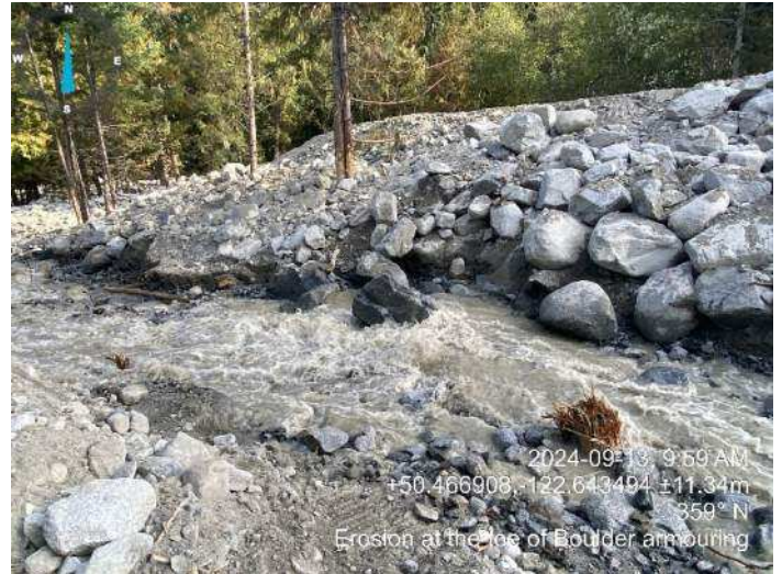
Image 11: erosion at the toe of the bank causing 1 boulder settle into the channel (2024-09-13 @ 9:59 AM)
