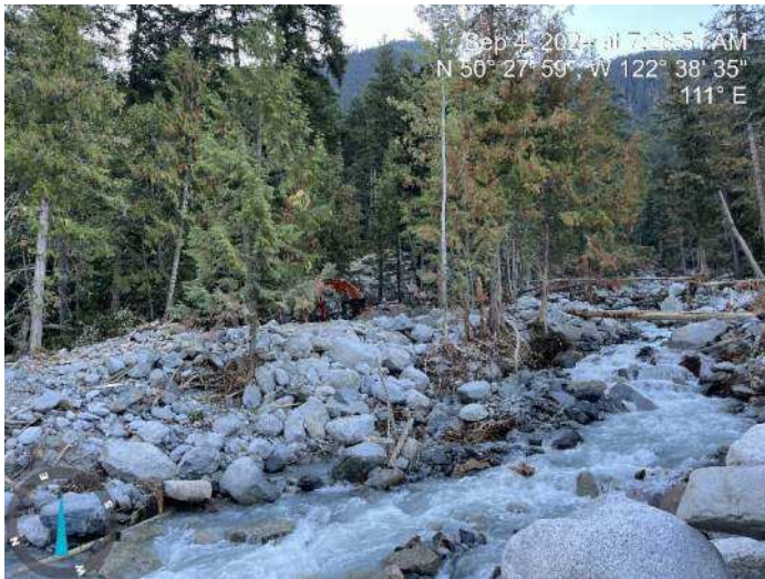
Image 2: 350 excavator continued to sort through materials from the debris flood deposits to build up the proposed embankment (2024-09-04 7:28 AM)
