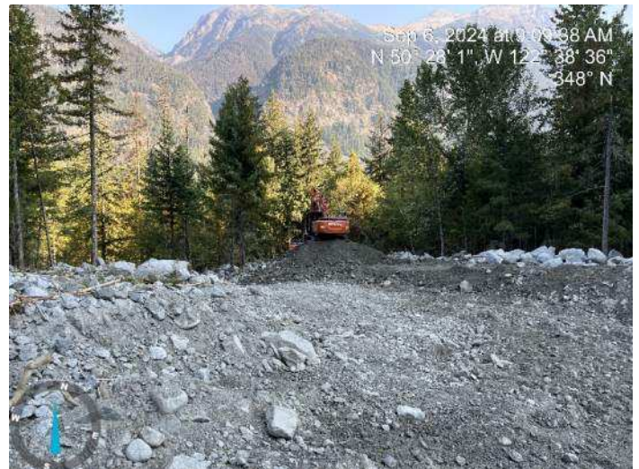
Image 5: 350 and 210 excavators working together to excavate proposed channel, and stockpile materials to build up the proposed embankment (2024-09-06 9:09 AM)
