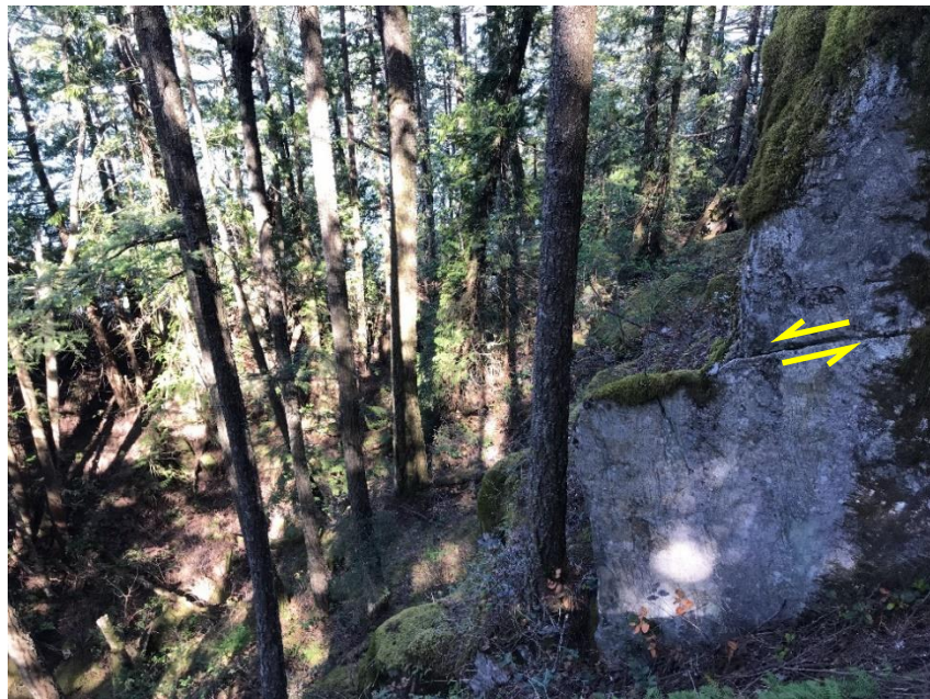
PHOTO 8: View of steep bedrock bluffs within the Northwest area. Yellow arrow indicates unfavourably oriented fracture plane dipping out of the slope. (Photo taken by Thurber in May 2019.)
